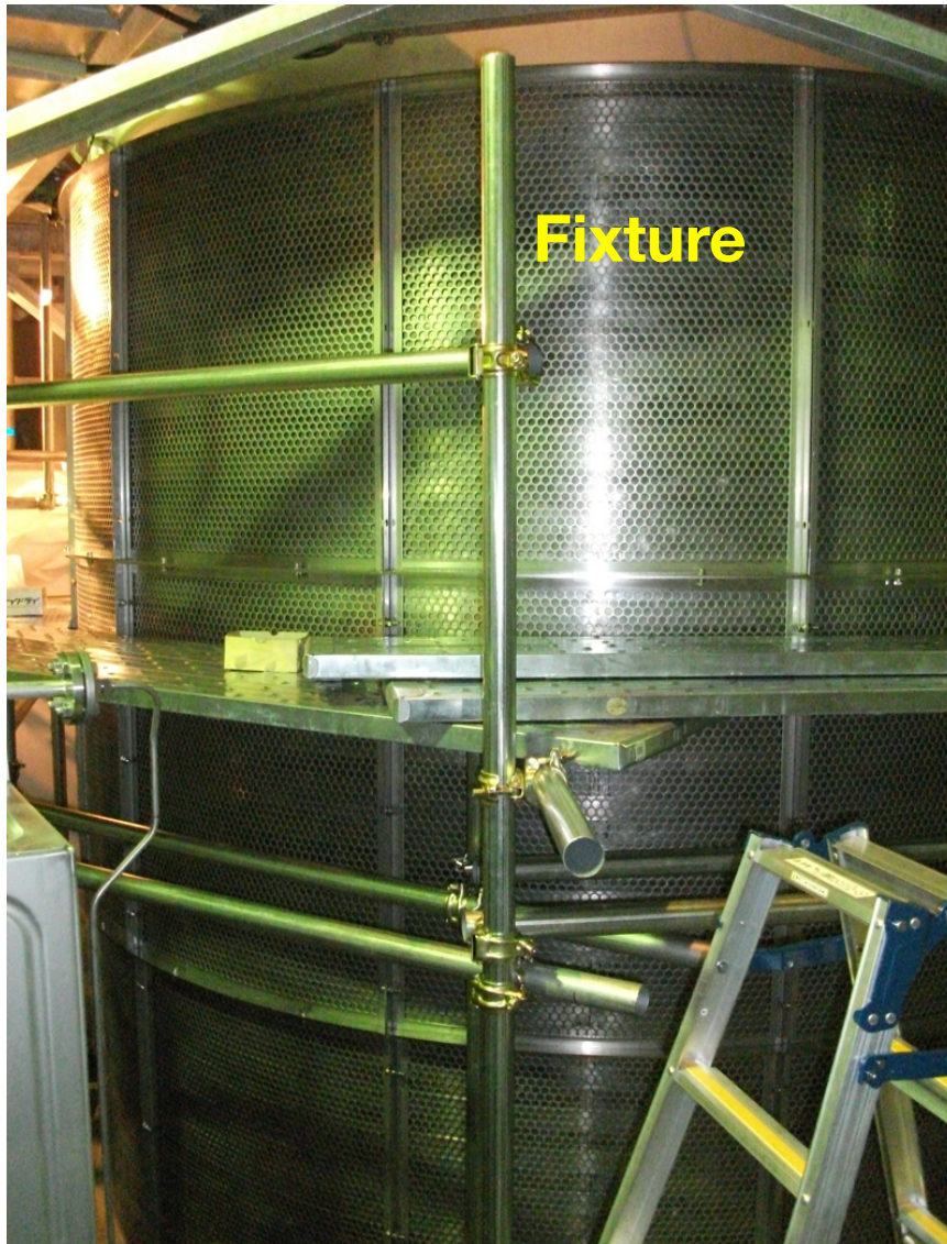
Side of stainless steel tank (Mar.17)
